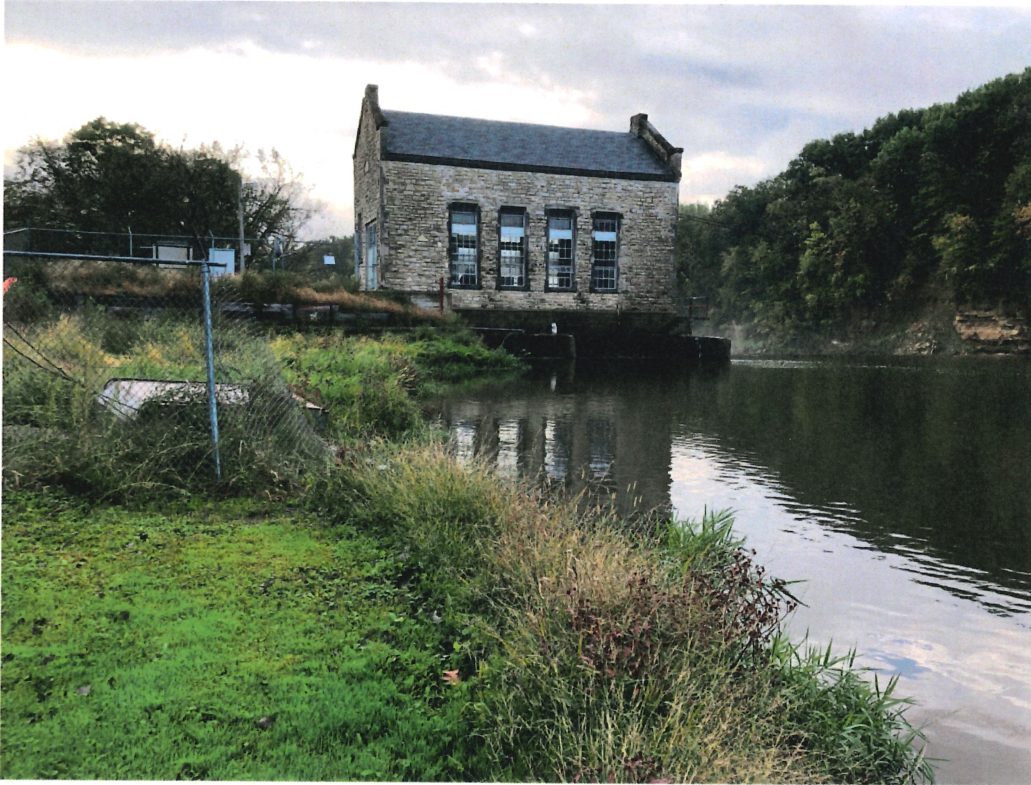
Figure 8: River Bank Erosion Near Dam, View 4
