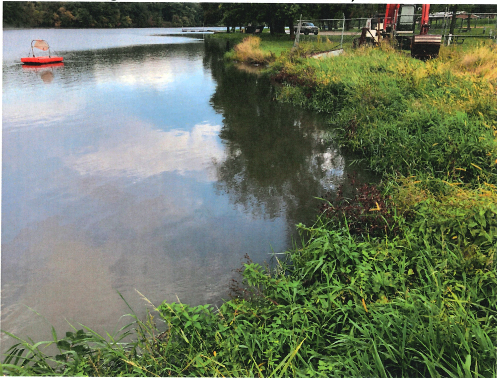
Figure 9: River Bank Erosion Near Dam, View 5
