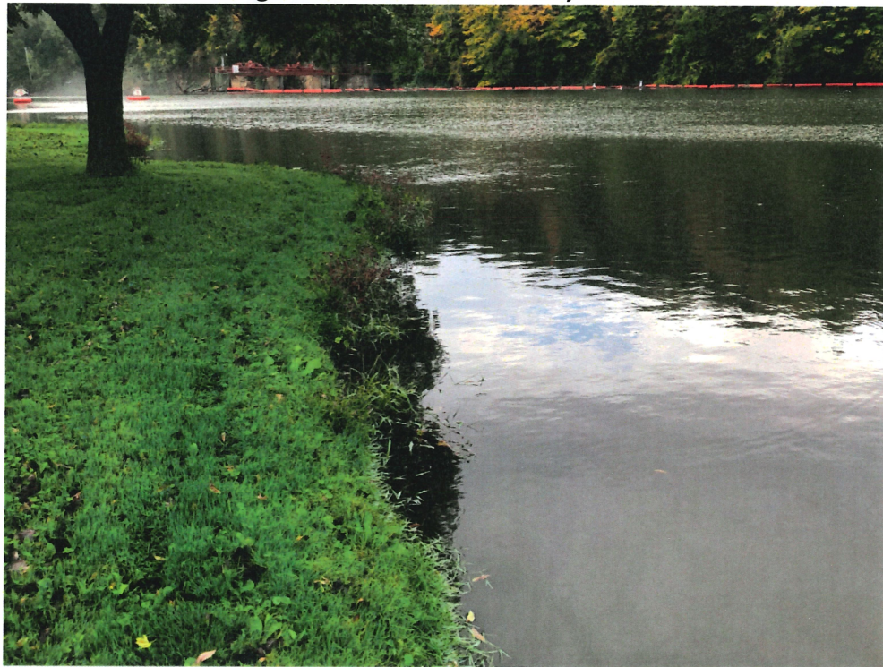
Figure 5: River Bank Erosion, View 1
